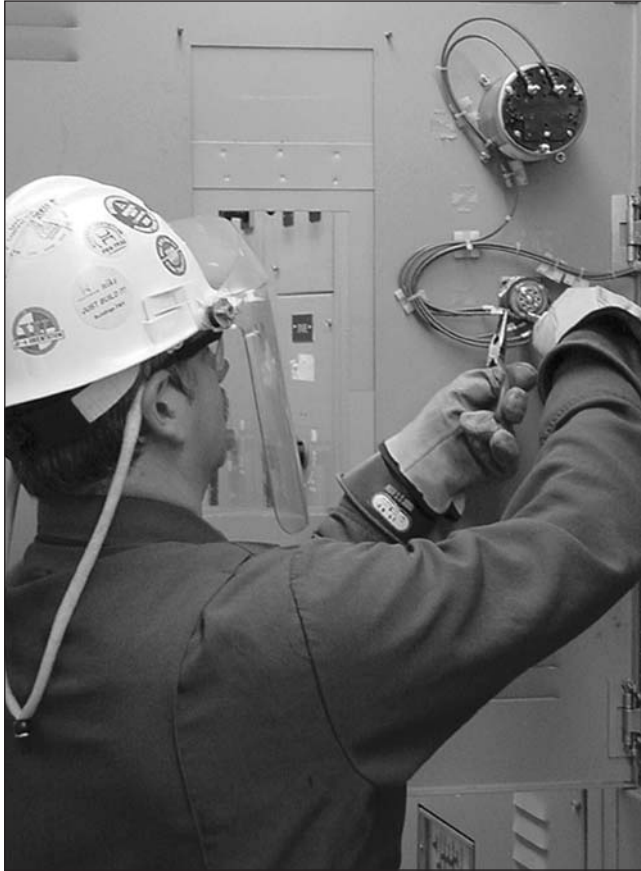
A workman with suitable personal protective equipment (PPE) working on energized equipment.
