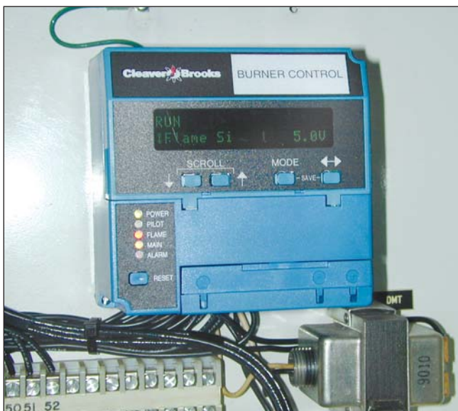
The BMS or burner management system is the brains that monitors/directs safe firing and operations.
