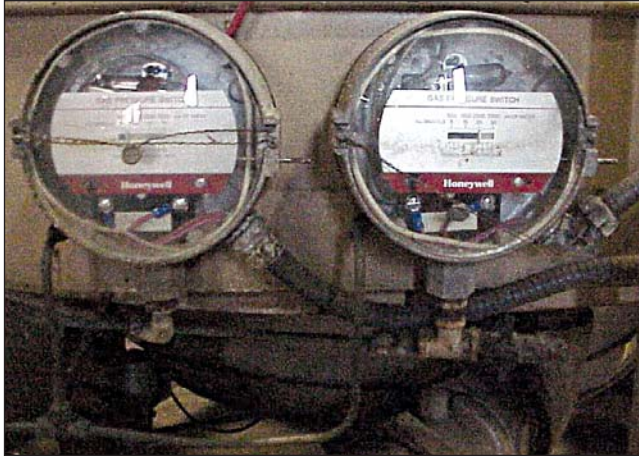
Typical high/low gas pressure switches to verify gas pressures are in the proper range.
