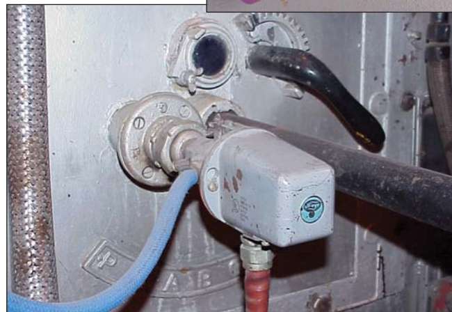
Typical flame scanners that monitor conditions.
