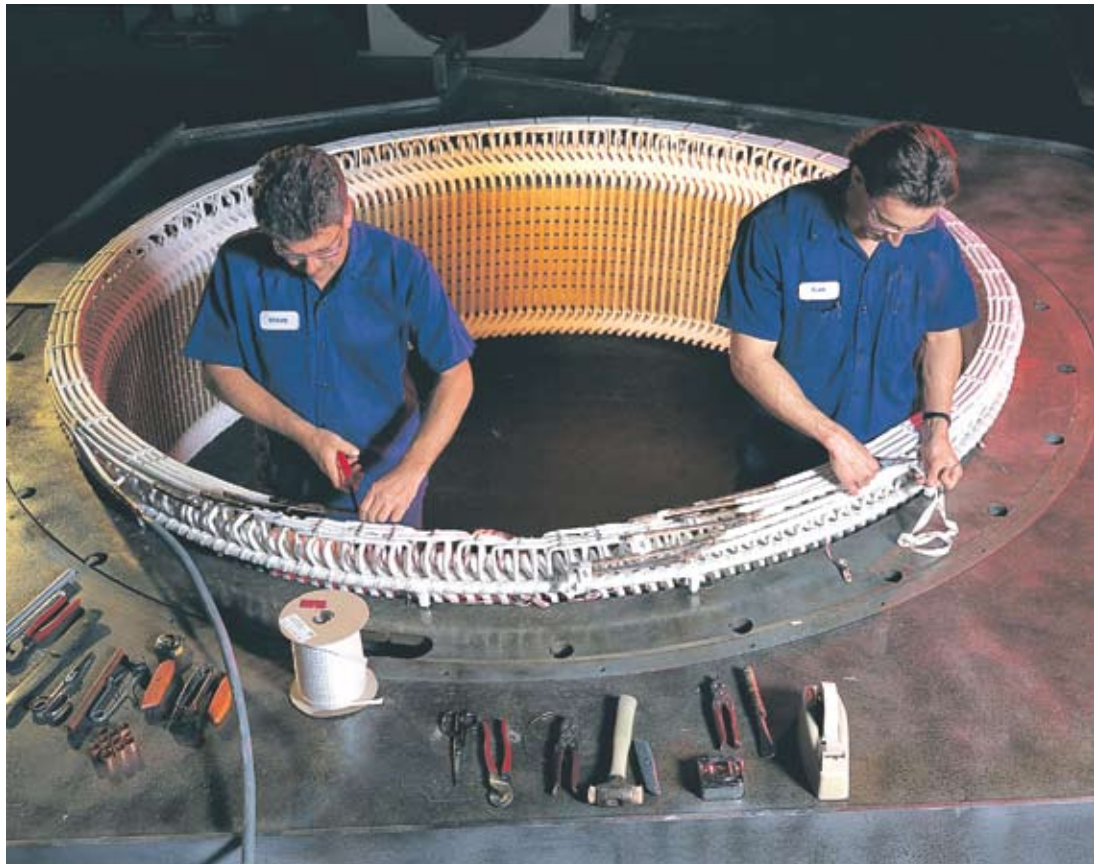
Figure 1. Tape provides both insulation and a substrate to which the varnish bonds.
